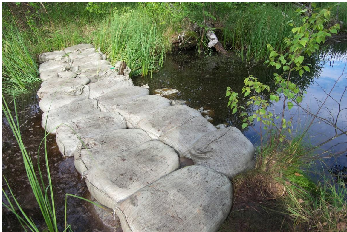
Figures 7 and 8. Two stages of the construction of dam in the branch of drainage channel in disturbed peatland Bolshoye Boloto.
