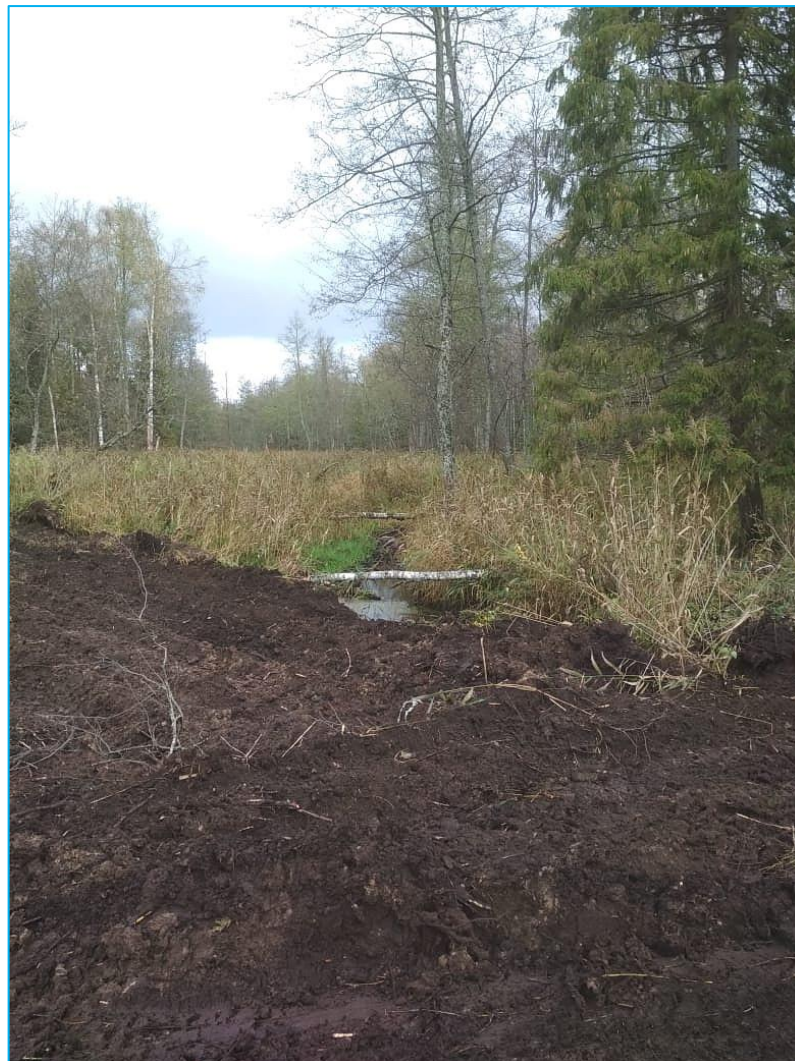
Figure 2. The dam on the drained ditch No. 4 in the process of construction.
