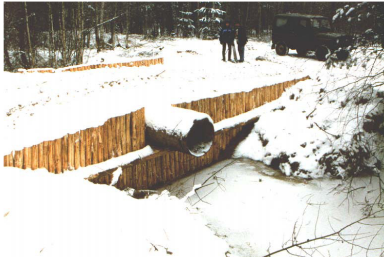
Fig. 20: A single dam, designed to double as a bridge, was installed in the canal collecting water from the ditches crossing the peat field (photo Ecological Centre Dront).
