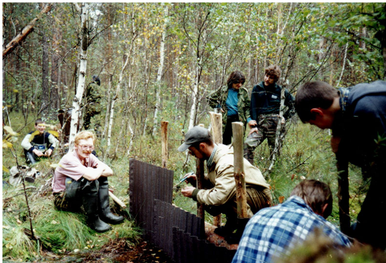
Fig. 21: Construction of dam from the corrugated plastic sheets (photo Taldom Administration of Specially Protected Nature Areas)
